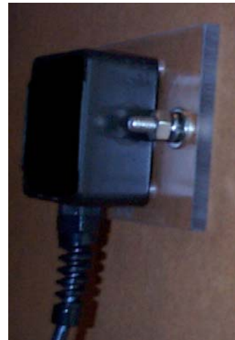
Figure 3. Display Interface Module Installed and Viewed from Inside of Field Equipment
